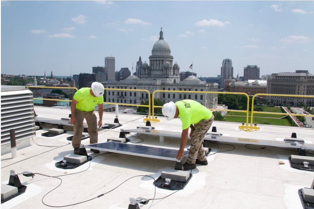
Powers Building, Capitol Hill Complex — 180 kW Solar PV Installation
