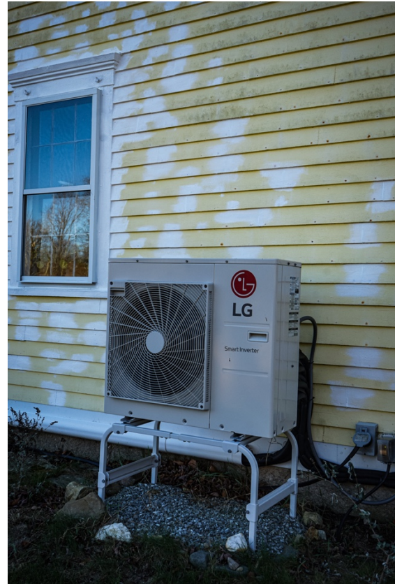
Outside system for air source heat pump at Burgess Farm
