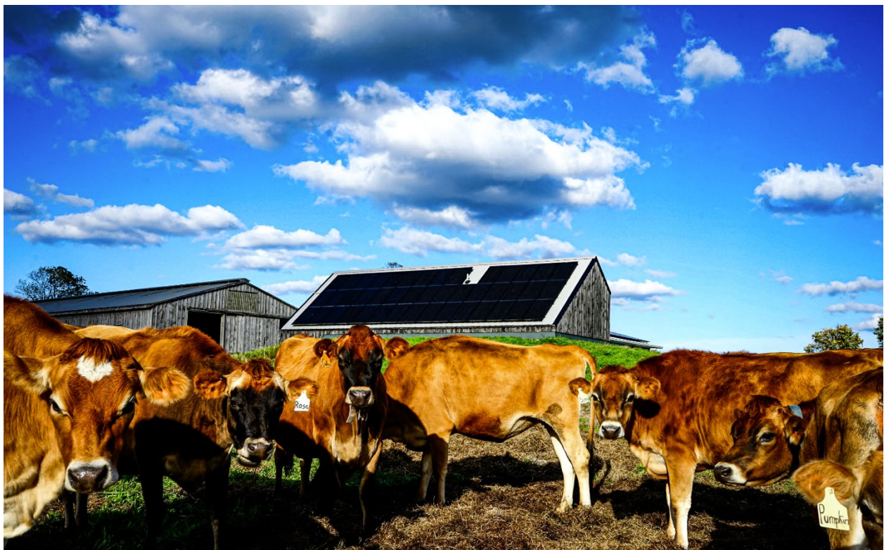
19.8 kW Rooftop PV System at Sweet and Salty Farm, Little Compton, RI
