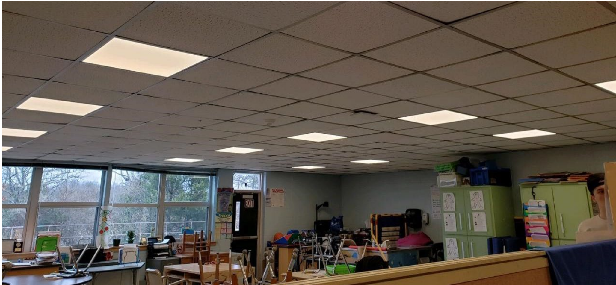
Lighting upgrade with LED and advanced control
