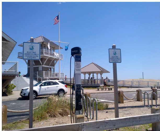
Figure 1: EVSE installation, East Matunuck State Beach
